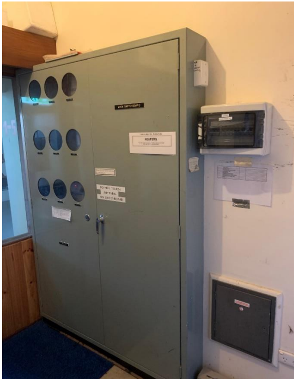
Main meter board
