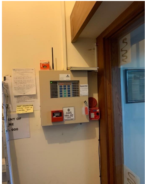
Fire control panel
