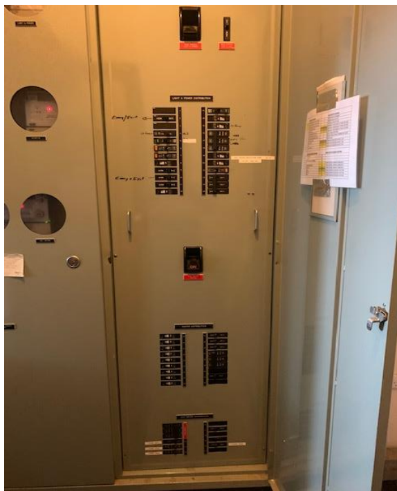
Main switchboard in central switchroom
