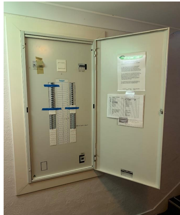
New wing sub-board
