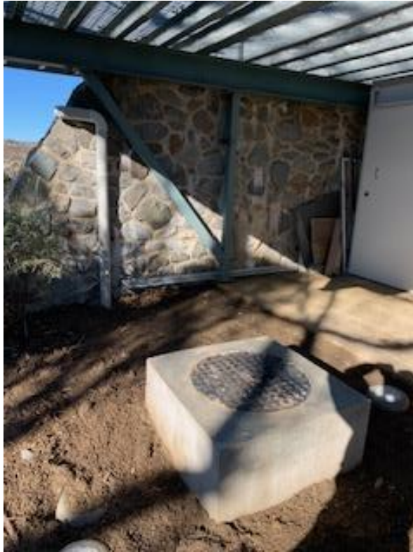
Grease trap on east side of south deck
