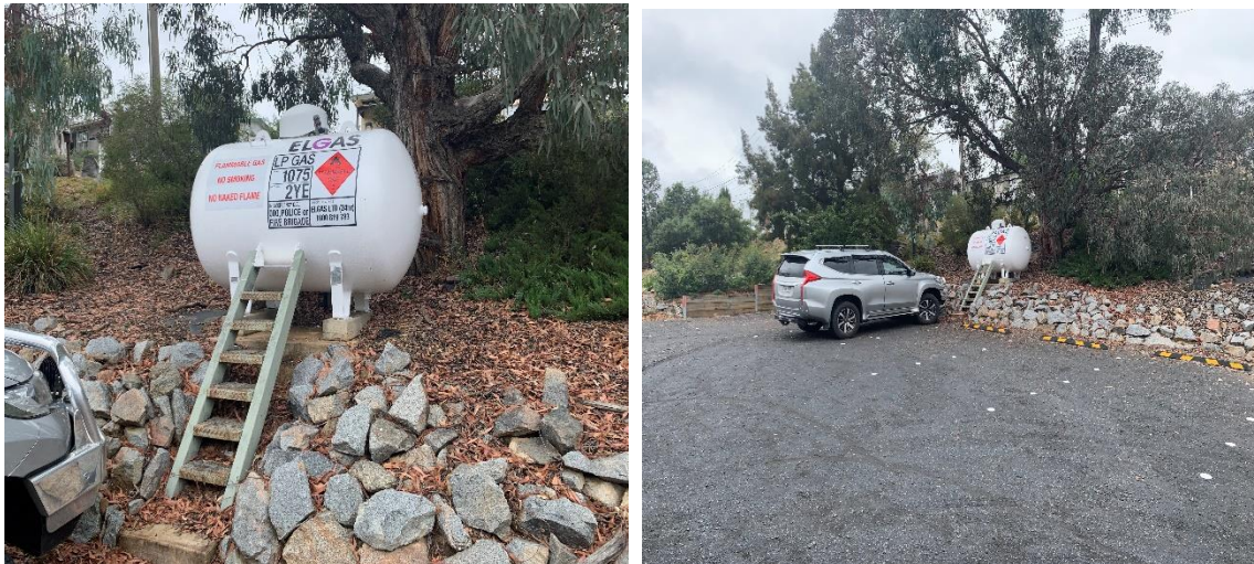
Main gas tank in car park
