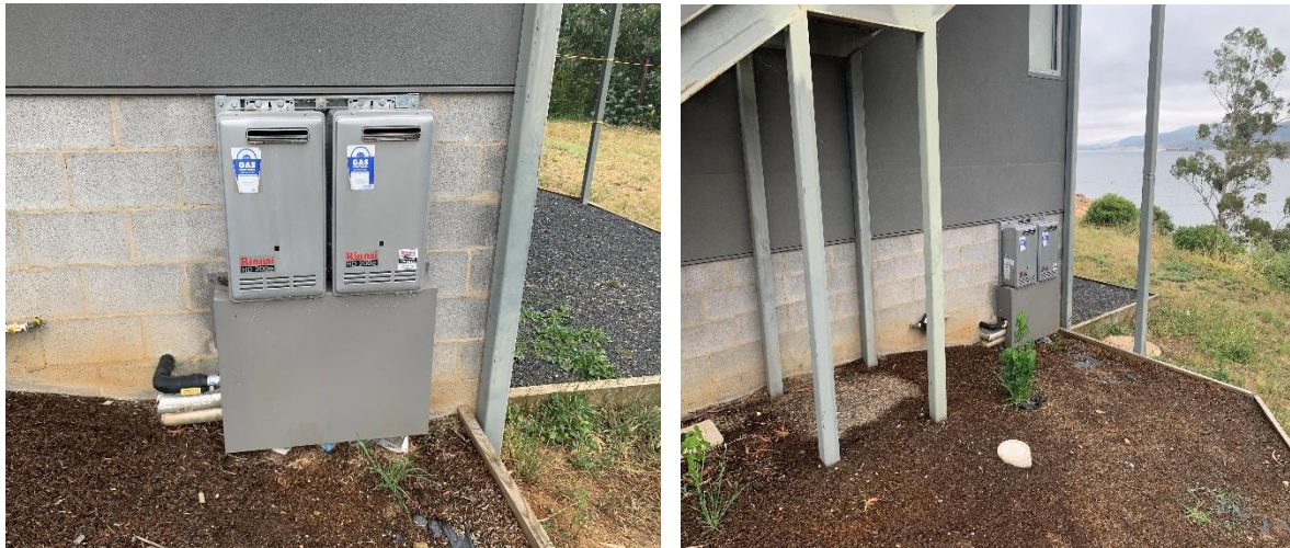
East wall HW gas heaters
