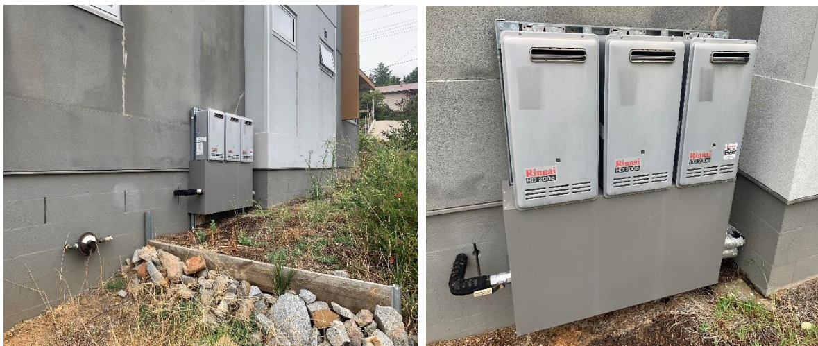
West wall HW gas heaters
